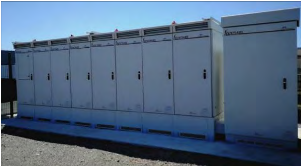
Plate 2.4 Typical outdoor centralised inverter
