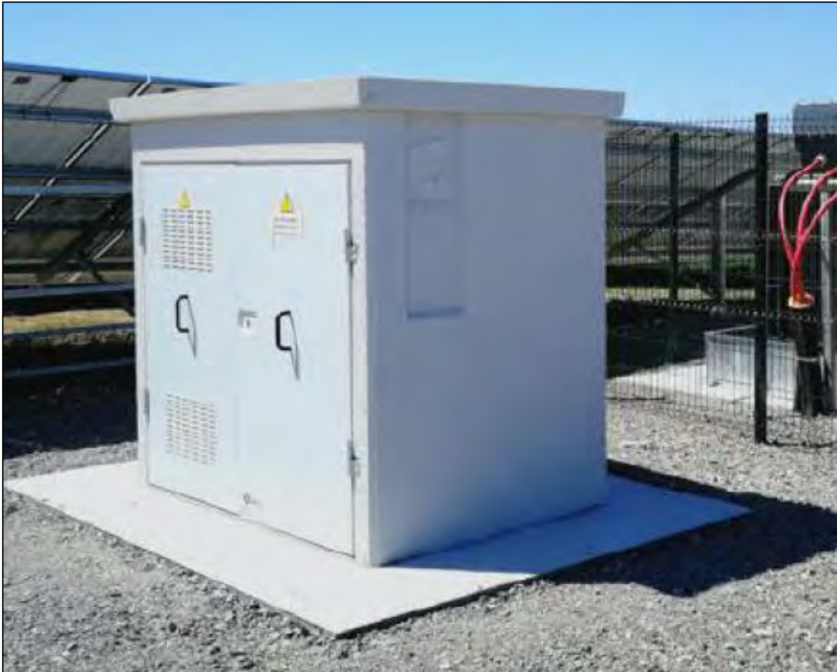
Plate 2.6 Typical outdoor switchgear
