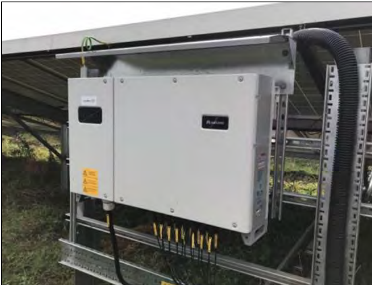
Plate 2.3 Typical string inverter
