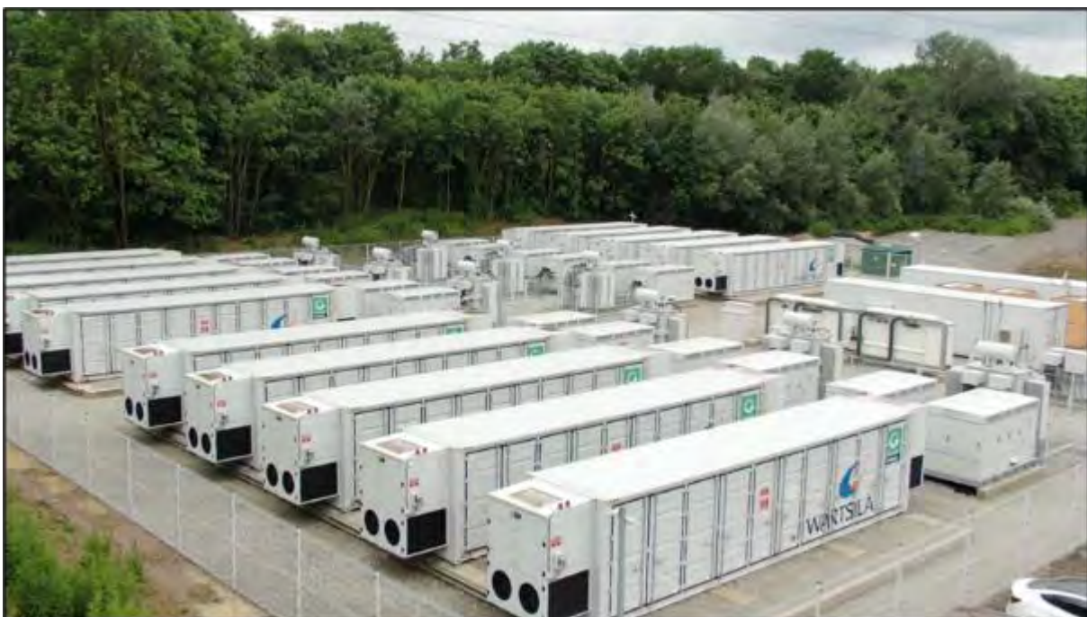
Plate 2.9 Example BESS facility
